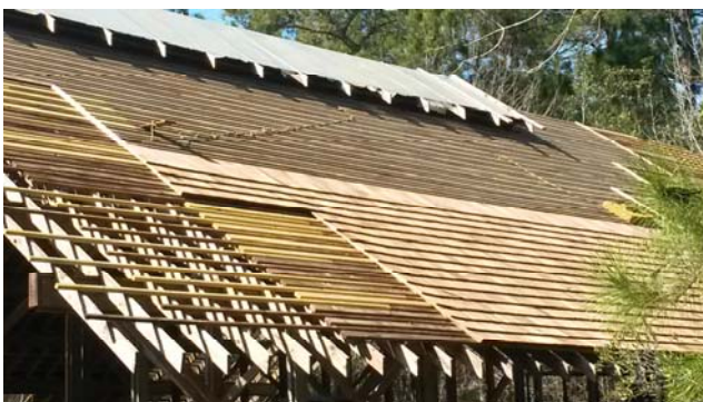
Remodeling of the Pinecote Pavilion is well underway. Shown above, the new roof installation in progress in February.
