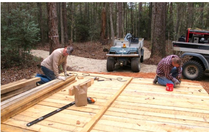
Volunteer Tom Heim and Terry Johnson work to install the cypress planking for the beautiful new deck located at the intersection of the Swamp Forest Trail and the Slough Trail .
